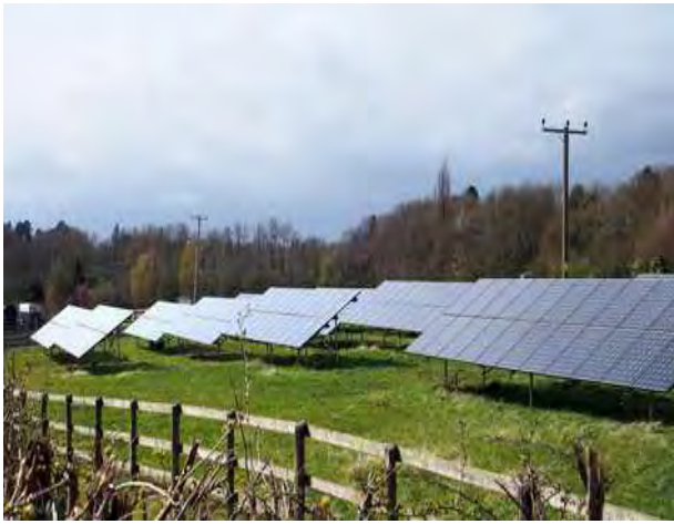
solar panels at Priors Court
