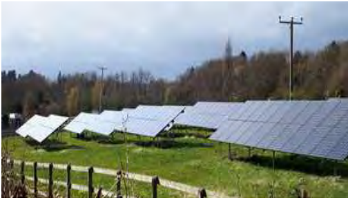
solar panels at Priors Court
