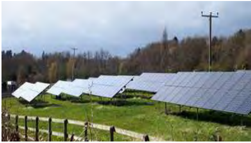
solar panels at Priors Court
