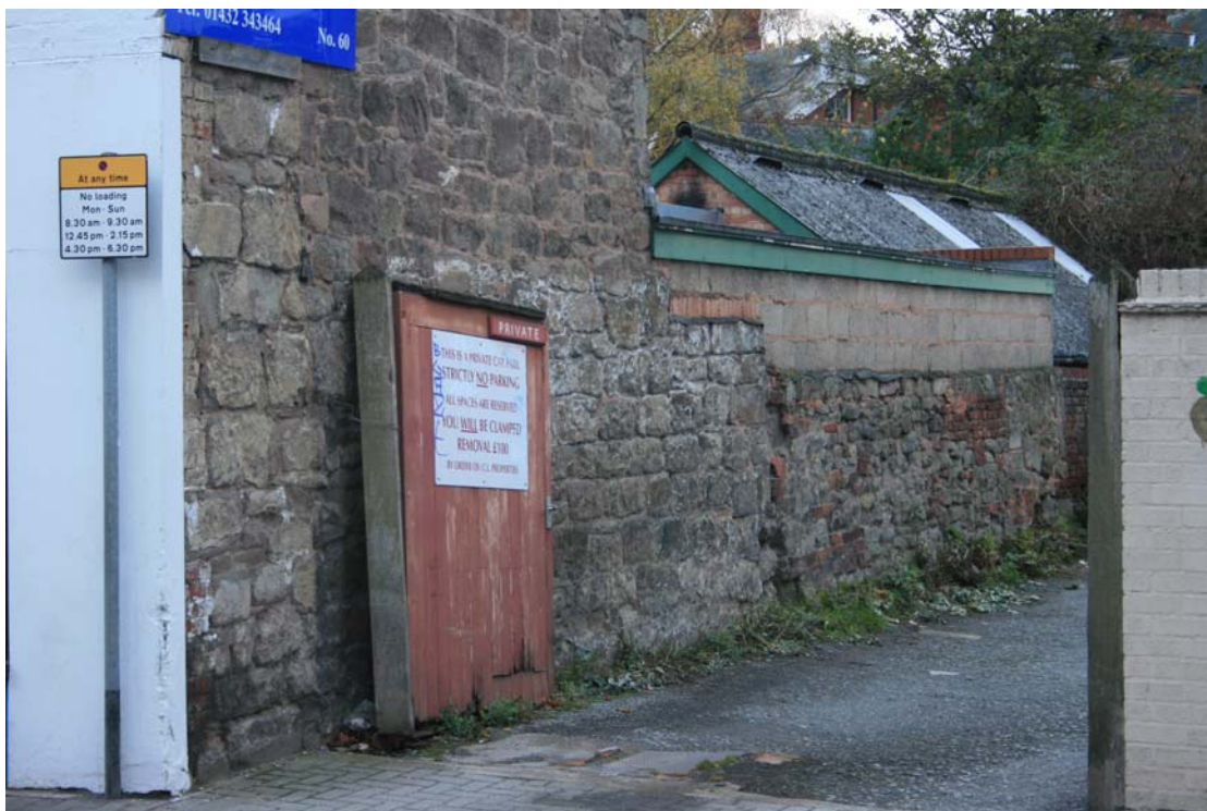
The city wall (inner face) on the south side of St Owen Street. There are clear differences between the ? primary masonry at ground-floor level, the upper floor of the frontage building, and the garden wall to the rear on the city wall line
