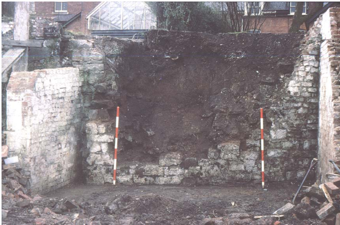
Photograph of the Mill Street – Cantilupe Street wall after removal of collapsed debris, immediately prior to excavation in 1972. (Photograph: Ron Shoesmith)
