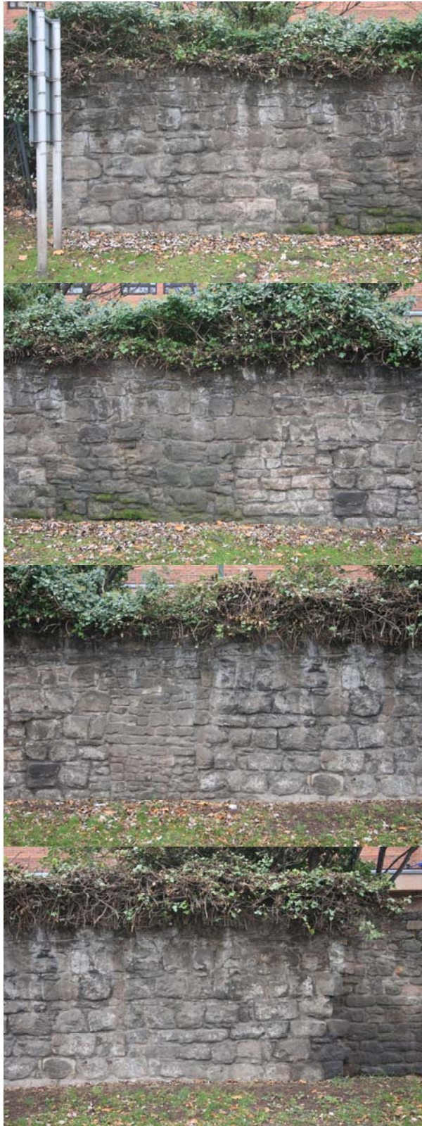
Sequential overlapping photographs of the outer face of the Maylord Orchards wall (western section) showing blocked openings in the primary type masonry. From east (top) to west (bottom). The last change in build shows the beginning of a set-back face, probably a repair in the 'SPAB' tradition
