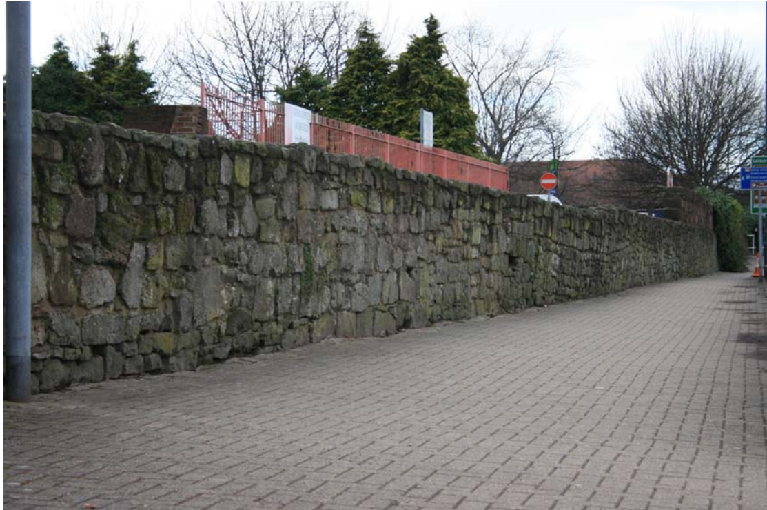
The Wall Street wall looking west alongside the New Market Street pedestrian underpass. The date of this masonry is unknown but is likely to represent a long history of ad hoc repairs in the post-medieval period with an uncertain degree of rebuilding c.1968; the blocks in the foreground may represent re-set primary facing masonry
