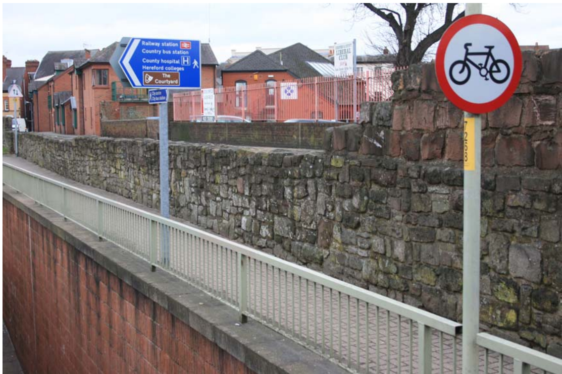
The Wall Street section, reduced in height alongside the pedestrian underpass. The eastern termination of the 1983 reproduction masonry is visible
