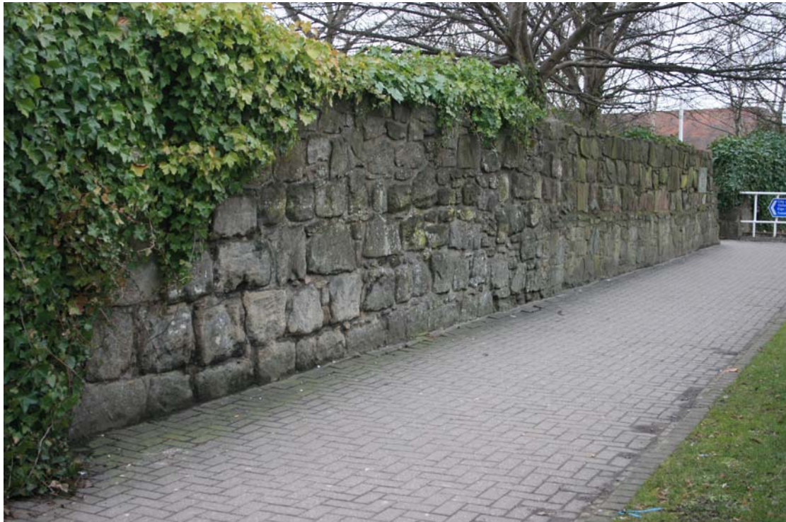
City wall masonry of probable 'primary' character (foreground), possibly as photographed above, to the east of the pedestrian entrance to the Tesco car park
