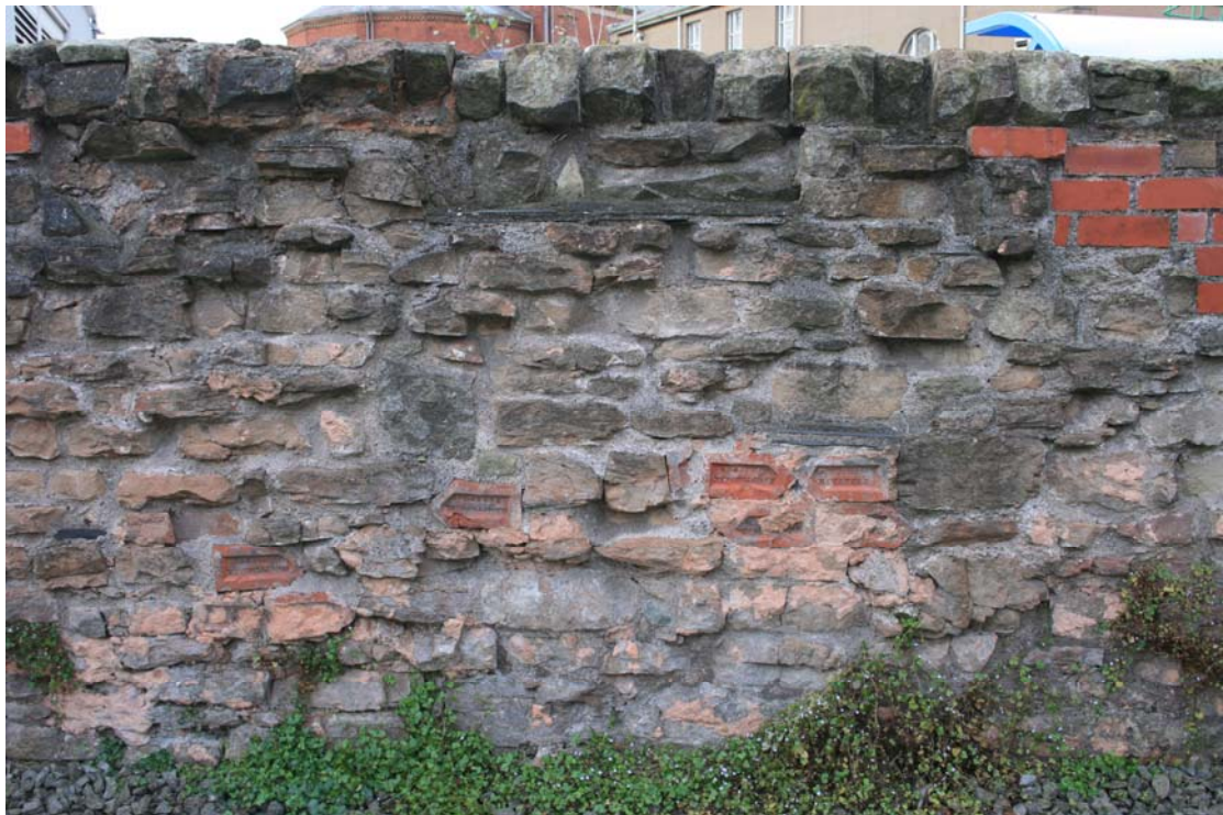
Detail of the rebuilt wall section making extensive use of 19 th -century brick at the rear of the car-park east of the Bath Street Police Station
