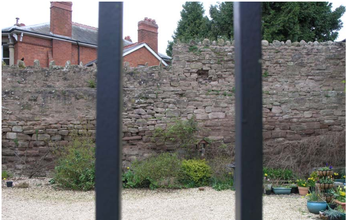
The wall in the garden of 14 Mill Street. The offset ledge marks the transition from the retaining wall to the garden wall on top. The condition of the wall in terms of missing and eroded stones, voids and lack of pointing is evident
