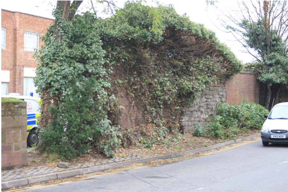
The inner face of the Maylord Orchards wall, looking east from the west end (2009). The problem of ivy, tree growth and the proximity of traffic to the wall face is apparent
