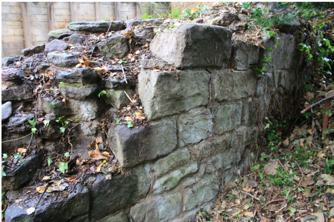
The city wall to the north of the entrance to the Cantilupe Street excavation. Excavation showed the face in this area to have been substantially rebuilt, possibly in the Civil War
