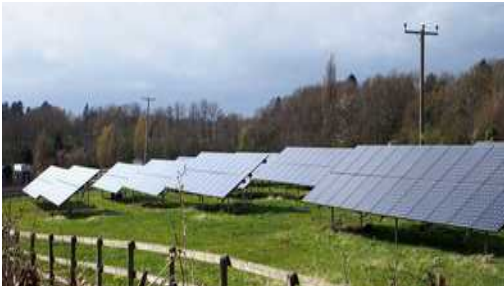
solar panels at Priors Court
