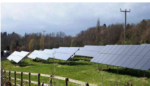
solar panels at Priors Court
