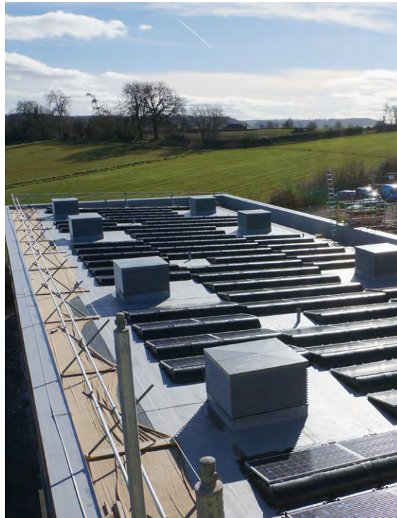
Fitting solar PV to our buildings is one way we can reduce our carbon footprint. The solar panels on Leominster Junior school are owned and operated by a community owned renewable energy co-operative 'Leominster Sunrise Co-operative' who provide reduced cost, zero carbon electricity to the school.
