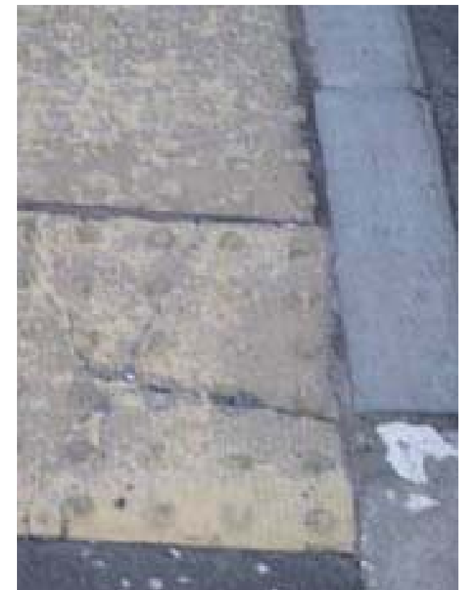
Example of typical cracked and faded tactile paving
