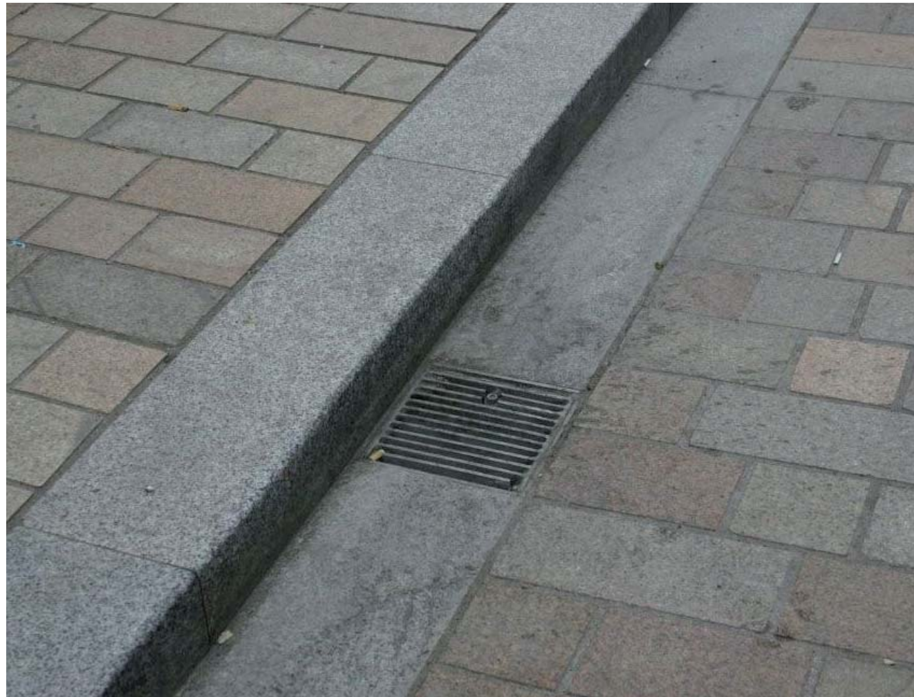
Simple, robust drainage details can help to remove water from the street and promote the quality of the streetscape
