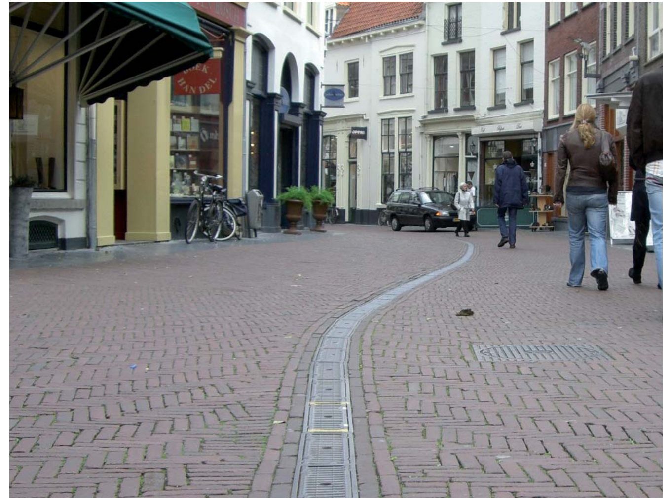
Drainage can also form part of the design of the street as a means of emphasising orientation and street geometry. (Zutphen, Netherlands)
