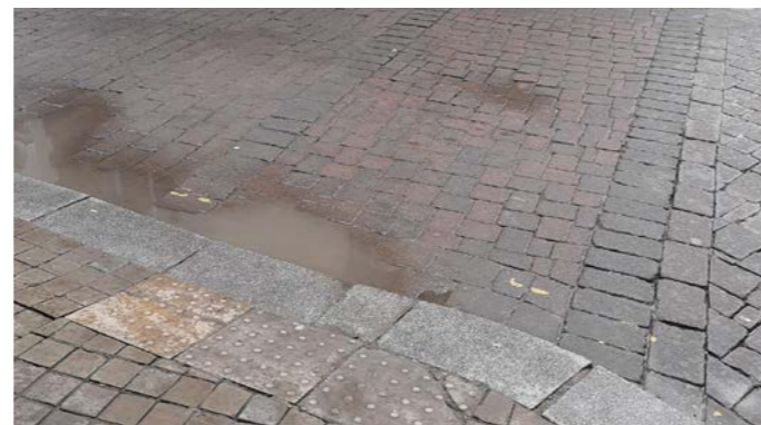
Poor paving surfaces and water puddling
