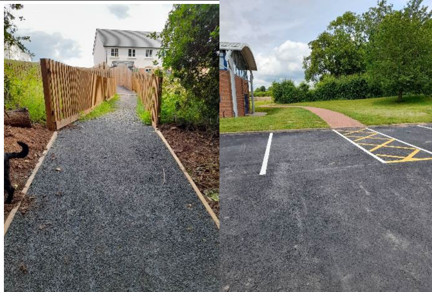
Figure 4 - Delivery of path through the copse to connect Vine Tree Close with Village Hall at Withington
