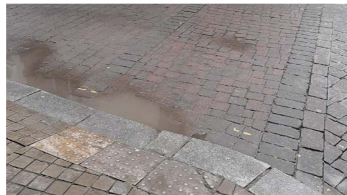
Poor paving surfaces and water puddling
