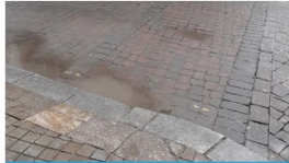
Poor paving surfaces and water puddling
