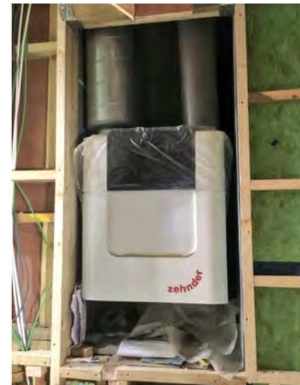
Image of Zehnder MVHR unit being retrofitted into an existing house (Source: Bow Tie Construction)
