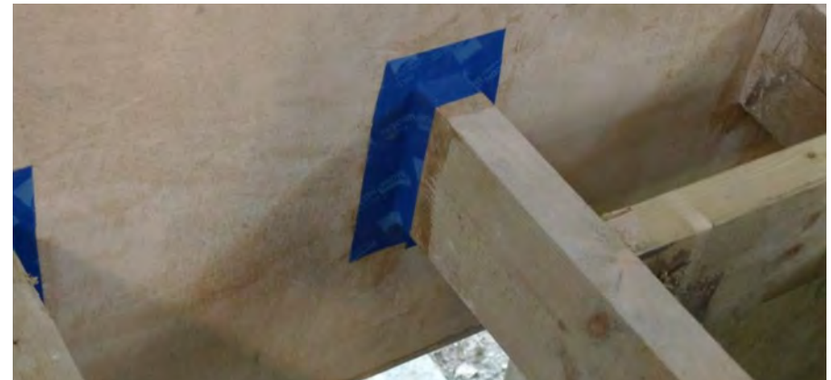
Applying airtightness tape to joist ends is a common measure required to achieve good airtightness in existing buildings. Large gaps may need filling with mortar first, and remember to apply a suitable primer. (Source: Ecomerchant)
