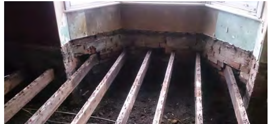
Achieving airtightness is possible in retrofit, but it is often necessary to strip back to the basic structure and perform basic repair work before methodically applying airtightness products and principles. Always consider risk of moisture and condensation. (Source: Eightpans)
