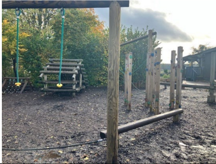
Figure 5 - Extension to staff toilet provisions, installation of outdoor playground equipment and IT Wi-Fi expansion at Canon Pyon Academy
