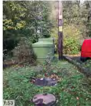
Figure 53: Utilities tank visible from the road erodes the rural streetscape character. New development should reduce visibility of utilities to maintain the character of the Neighbourhood Area.
