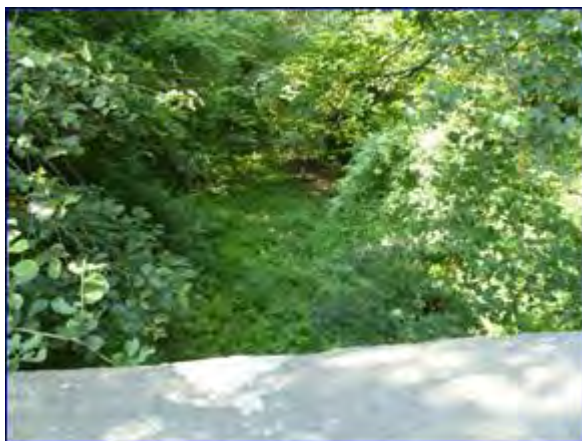
Figure 16 Overgrown Rail Alignment at Holme Lacy
