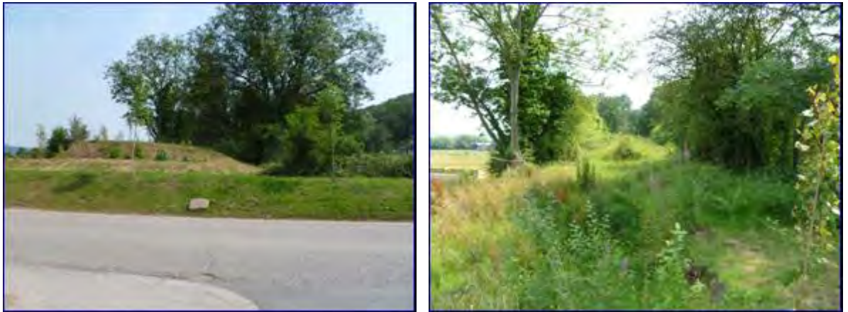
Figures 10 & 11 Embankment at Fordshill Road and overgrown formation
