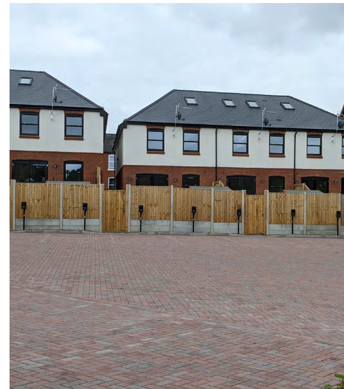
EV Chargers installed at a new development in Hereford.
