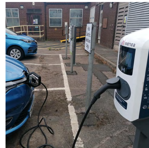
One of Herefordshire Council's electric pool cars being charged using the fast EV chargers at Plough Lane.
