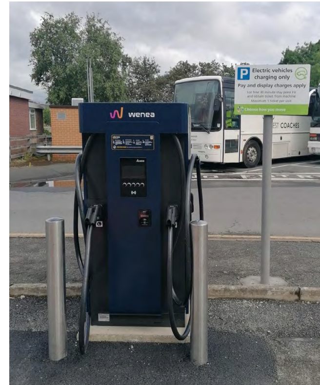
A newly installed ultra-rapid EV charging point at Broad Street car park, Leominster.
