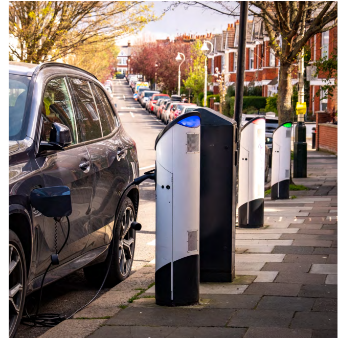
On-street EV chargers installed in other parts of the UK.
