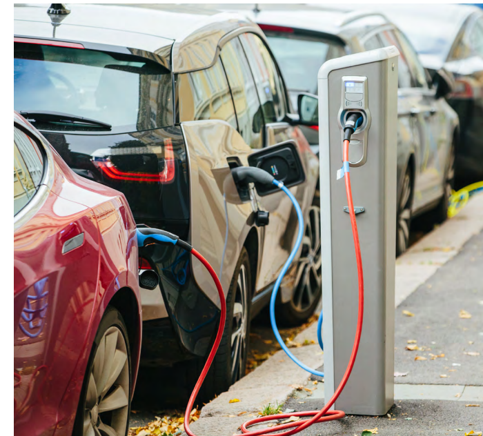
On-street EV chargers installed in other parts of the UK.
