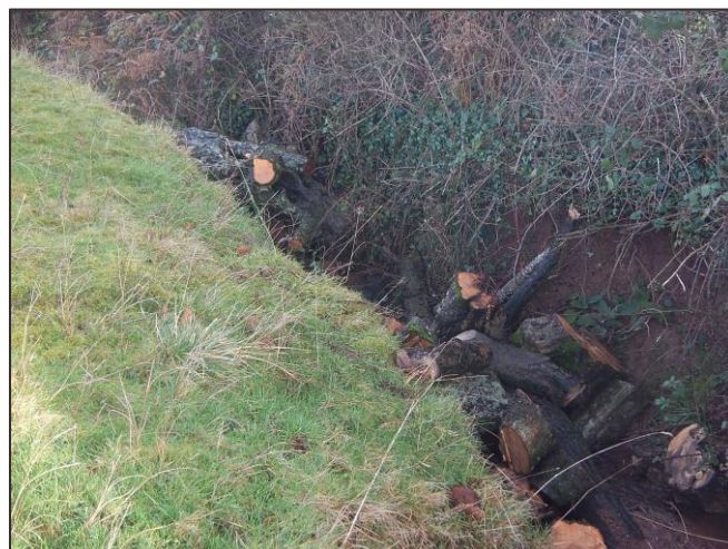
FIGURE 2 IN-DITCH SEEPAGE BARRIER SLOWING THE FLOW AT JAMIE'S FARM
