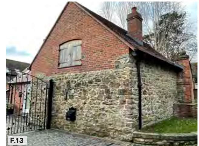
Figure 13: An example of stone and brick, a mix commonly seen where older buildings have been extended or modified.
