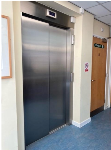
Image of lift on the ground floor
