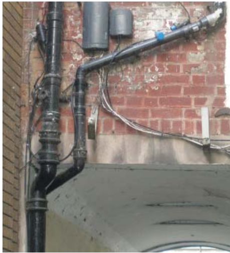
Untidy wiring and electrical boxes
