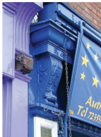
Surface mounted sign which partly conceals historic details
