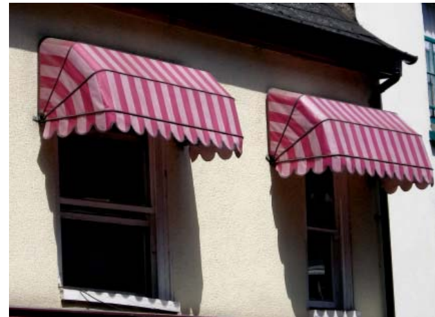
Dutch blinds are generally not acceptable
