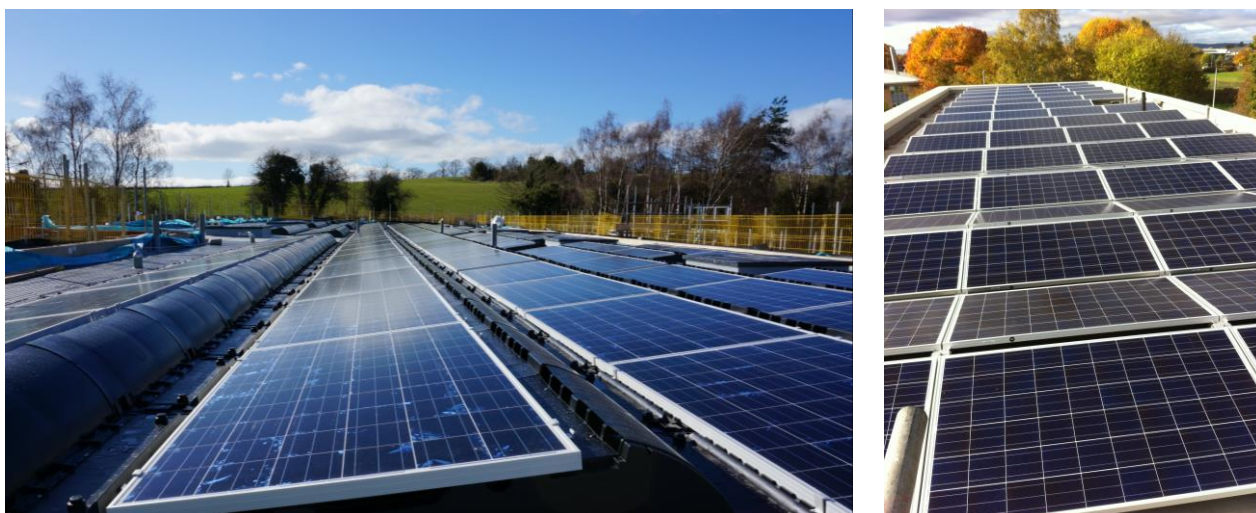
Figure 15: Solar photovoltaic arrays from around the County.
